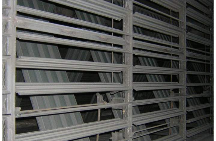
Air dampers like these need to be checked as part of a freeze rounds routine. BMS data isn't always accurate.
